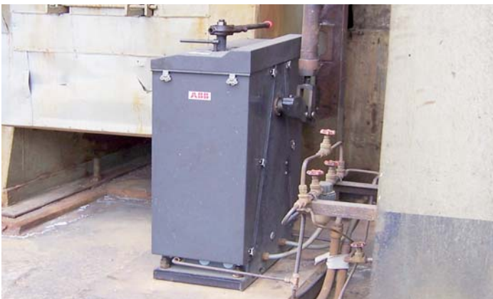
UP4 pneumatic rotary actuator on induced draft fan damper control
