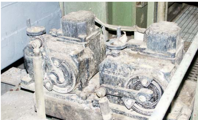
Actuator in burner air control
