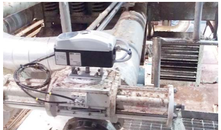
The EDP300 in a remote sensor installation
