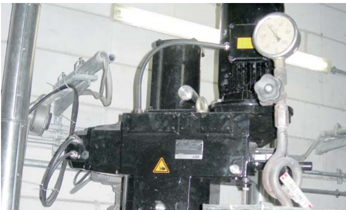
Actuator in high pressure desuperheater control
