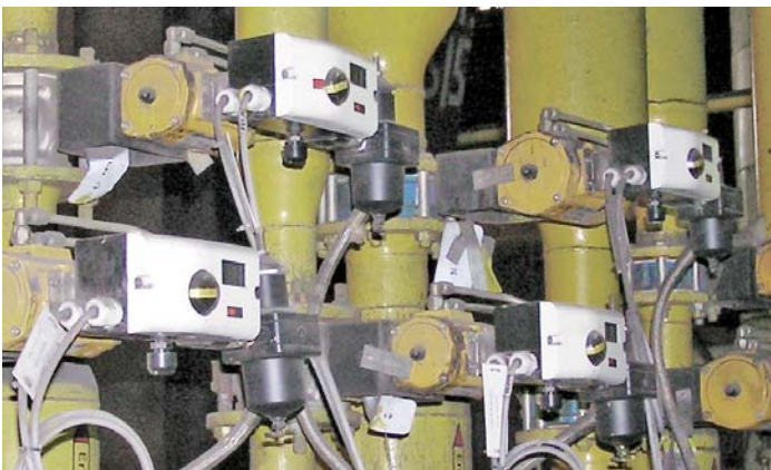
Digital positioners in a gas distribution station
